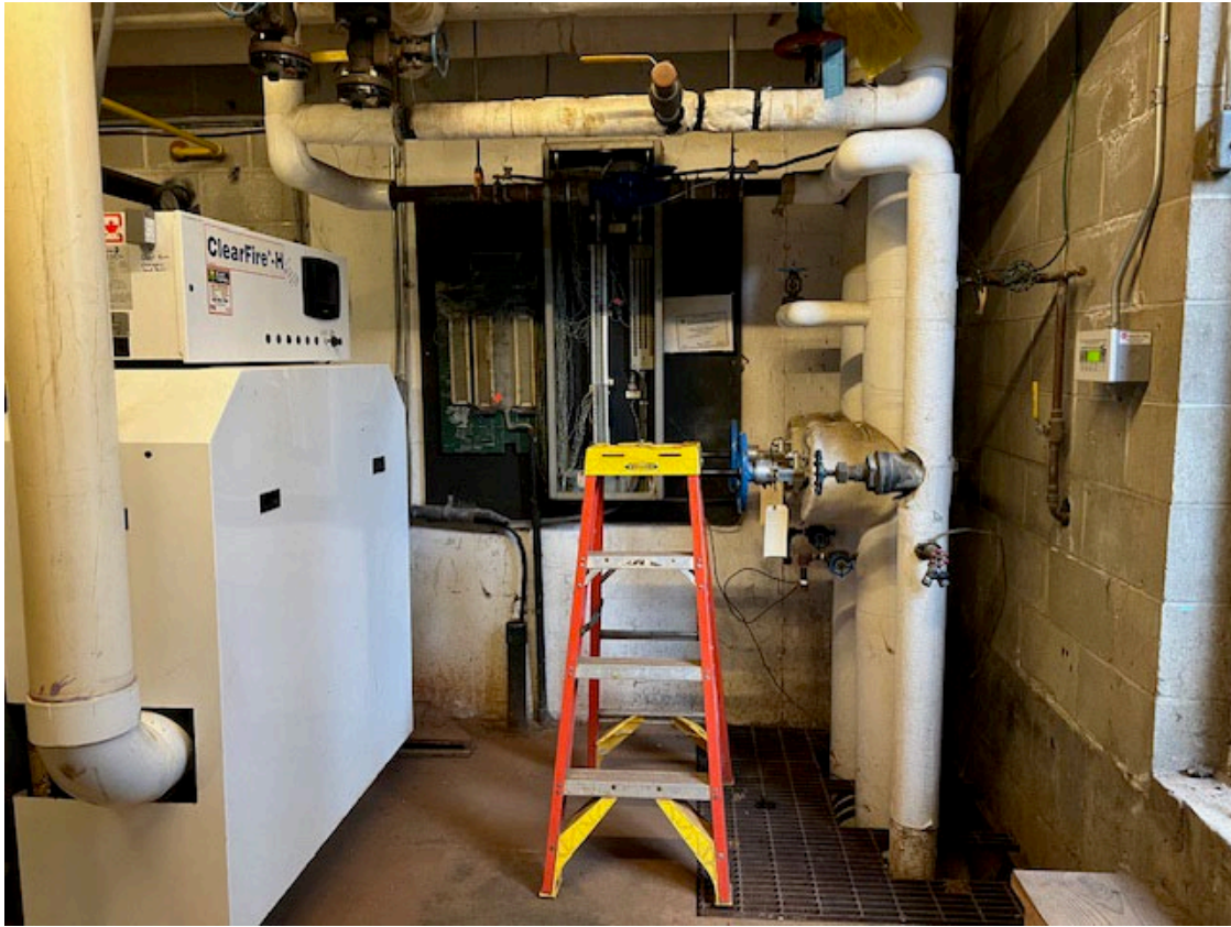
Interior views of Mech/Elec Room
