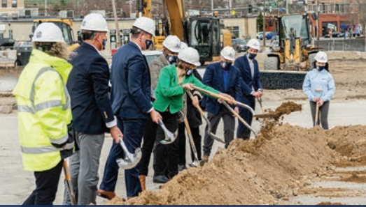
Campus and community leaders kick off historic construction project on USM's Portland campus.
